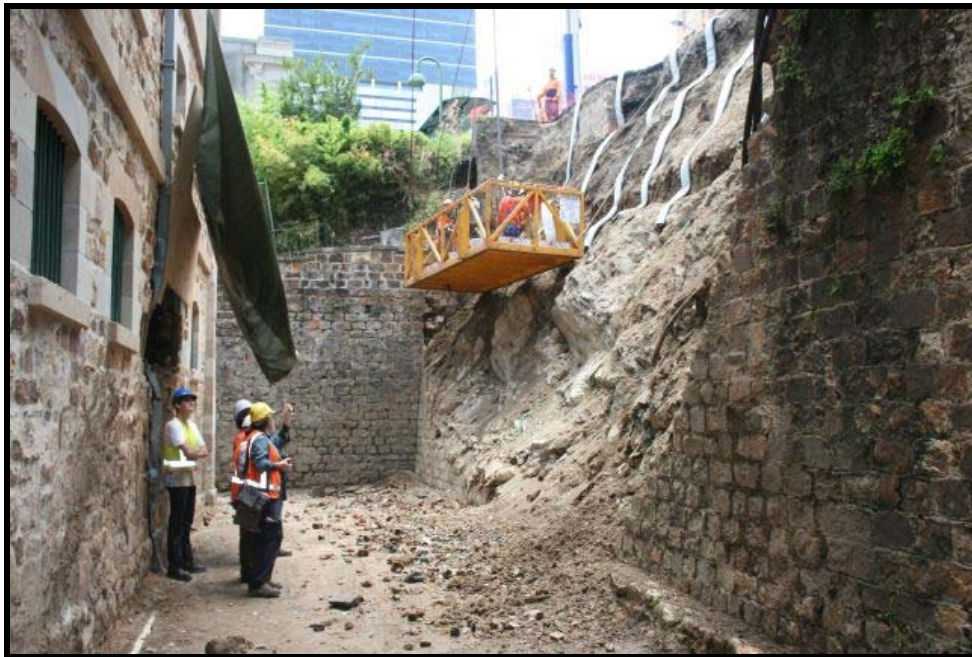
View west across the rear of the Commissariat Stores site showing extent of retaining wall collapse and efforts to restabilise the embankment (Source: DERM).
