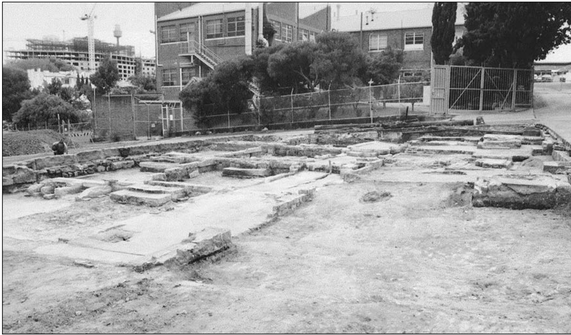
Fig. 4: View to southeast over the house and yard footings in Area A. House 15 is left foreground. Area following removal of demolition but prior to the excavation of the underfloor deposits.
